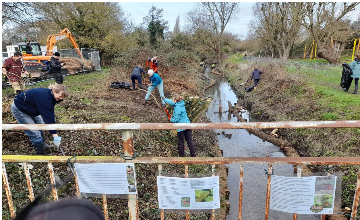
Restoration work on the East Cambridge Main Drain/Coldham's Brook near Abbey Pool
